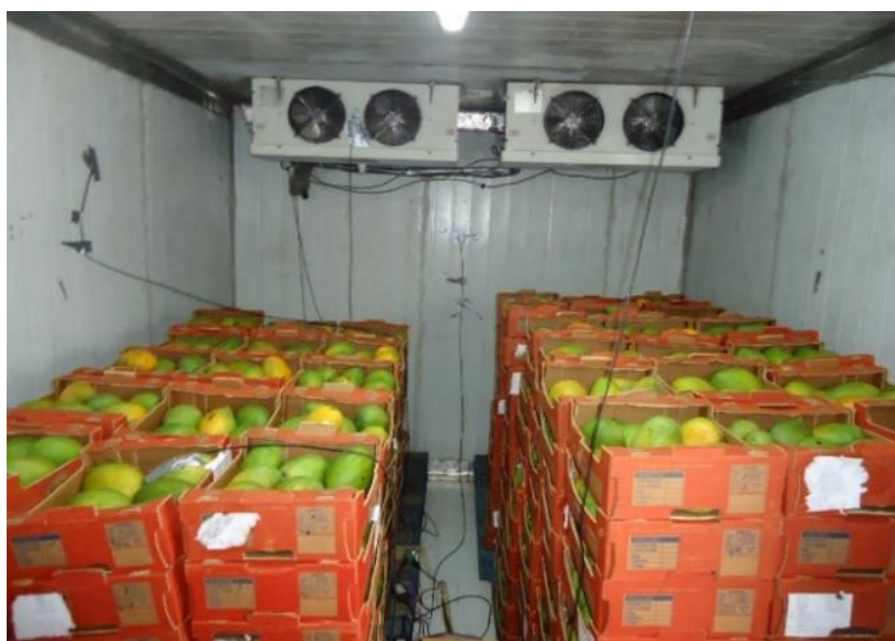
Fig. 1. Overview of the interior of the storage room with mangoes
